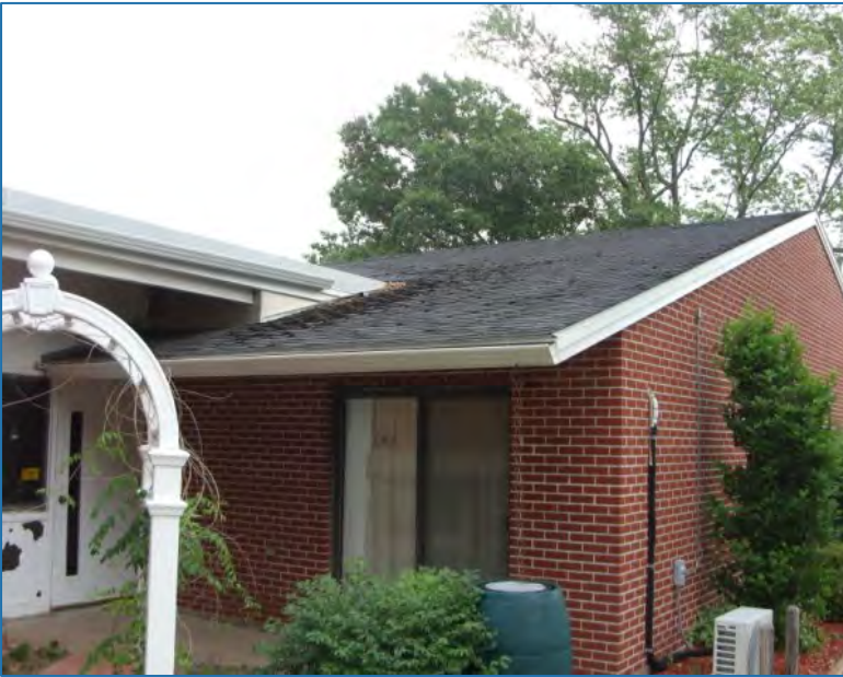
Plainfield UMC's loan helped with several building repairs, including these curling shingles
